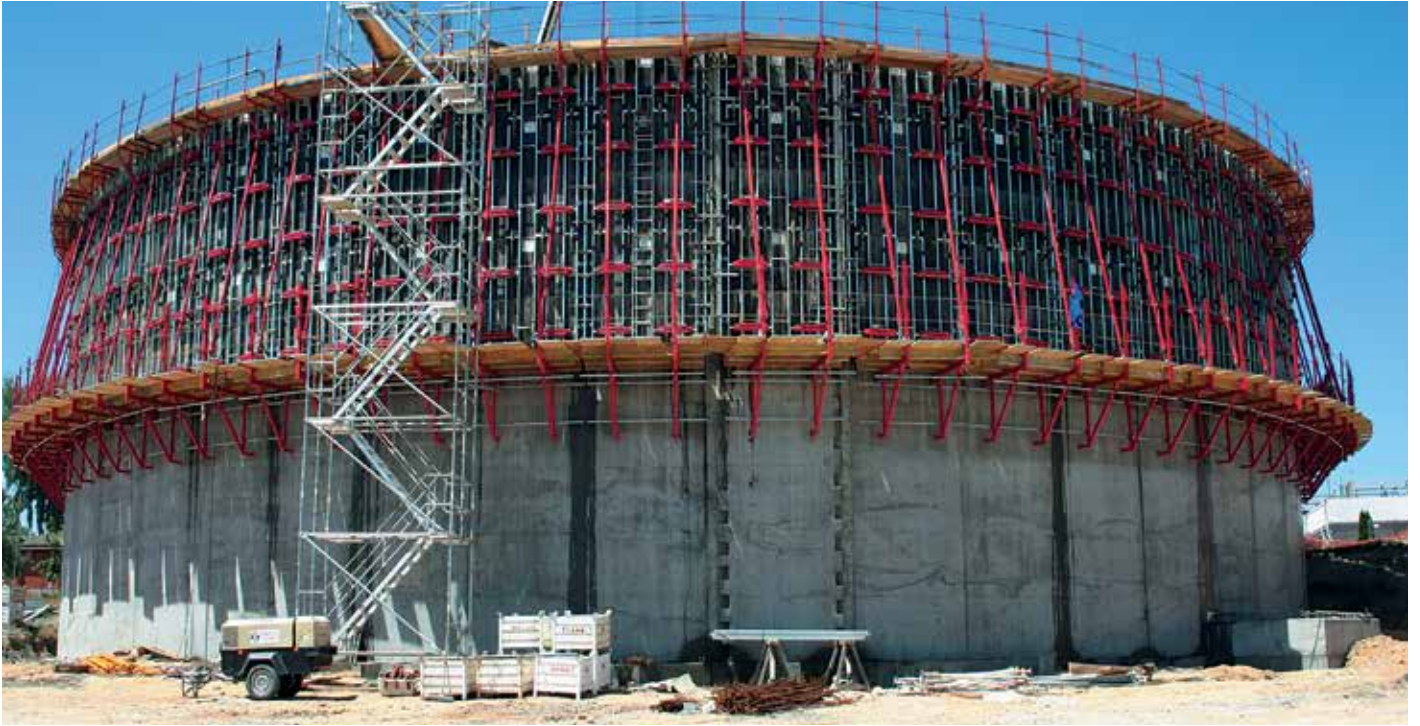
Waste Water Treatment Plant in Toledo, Spain
