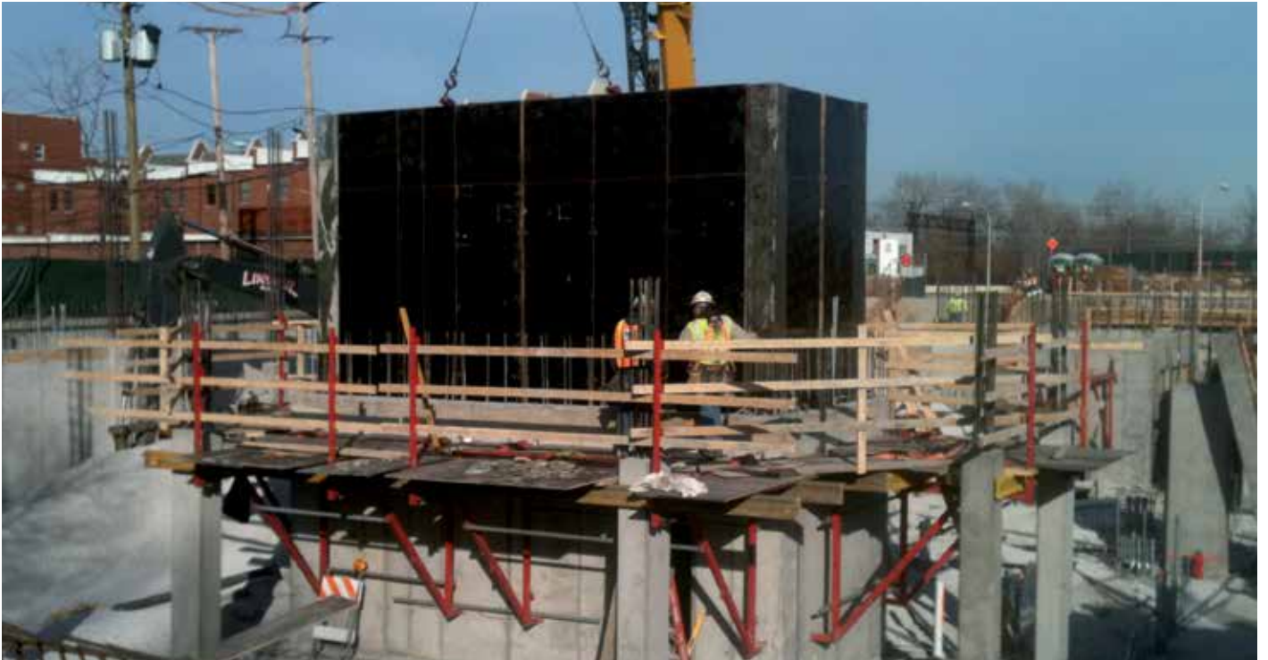
Lakepark Crescent Residential, United States
