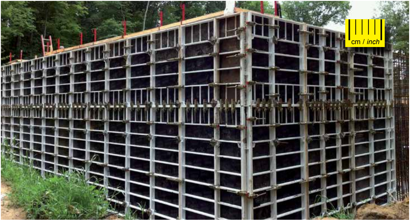
Koontz Lake Waste Water Treatment Plant, United States
