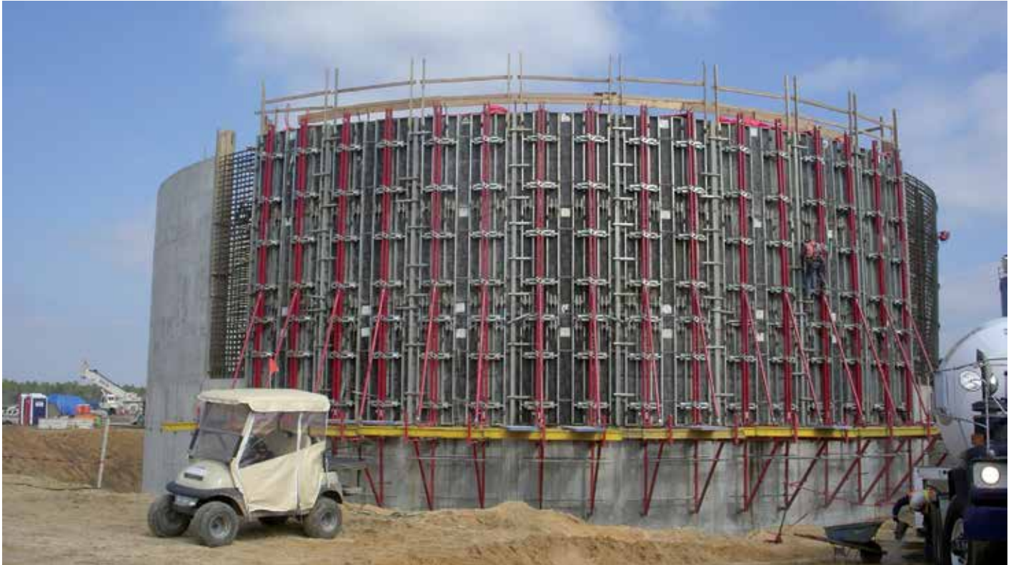
Thomas P. Smith Waste Water Treatment Plant, United States
